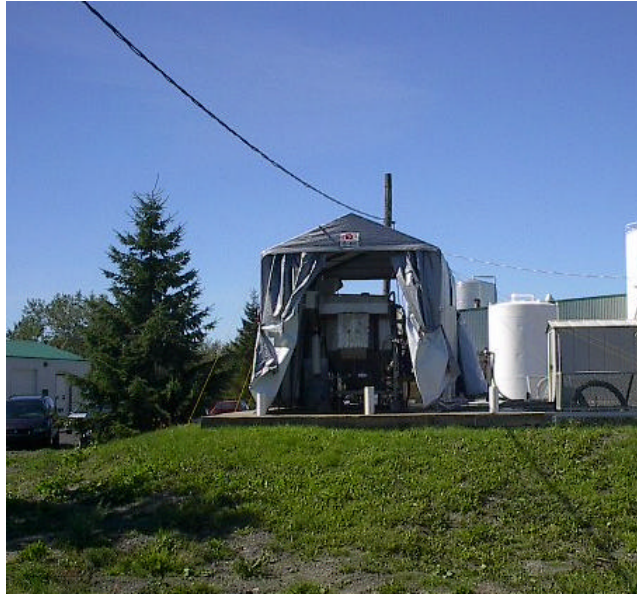
Mobile Unit installed at a Cheese Dairy
